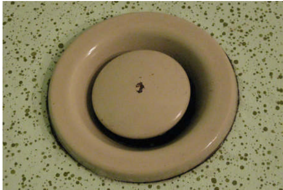
Ventilationsdon i badrum
